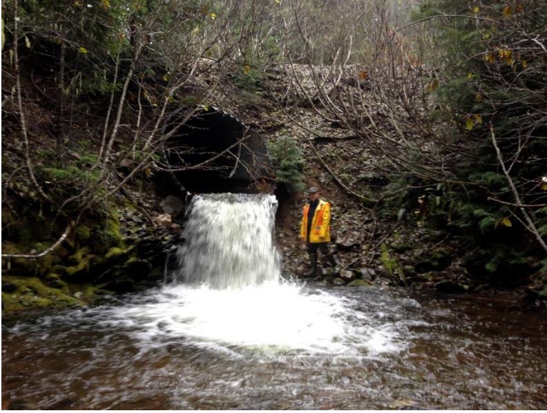
Picture 28. Impassable barrier at Granite Creek caused by culvert under FR1800. This barrier is considered repairable so the habitat upstream of it was included in calculations of stream habitat available to fish coming from Bumping Reservoir.
