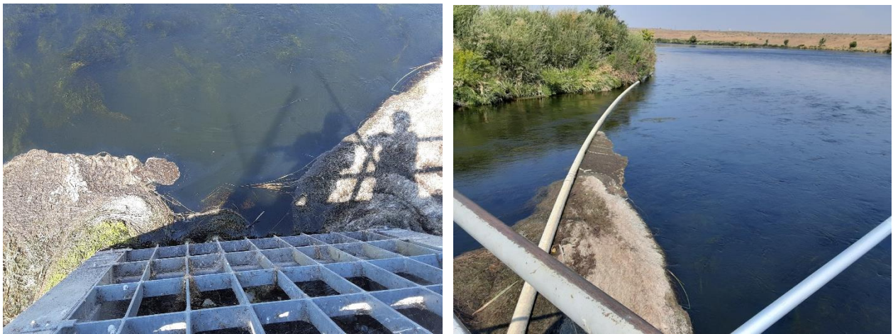
Figure 18. WSG mats impacting fish ladder gates, irrigation gates and overall dam operations. These structures are designed for larger wood material and require constant maintenance by BOR.
