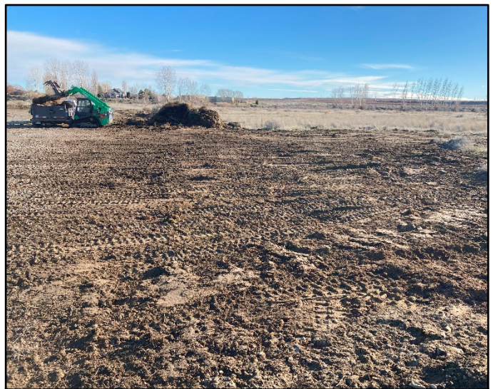
Figure 8. Removal of stargrass using a skid loader with grapple bucket attachment and dump trailer. The disturbed soil was re-seeded with native grasses the following week. Photo Credit: BCD
